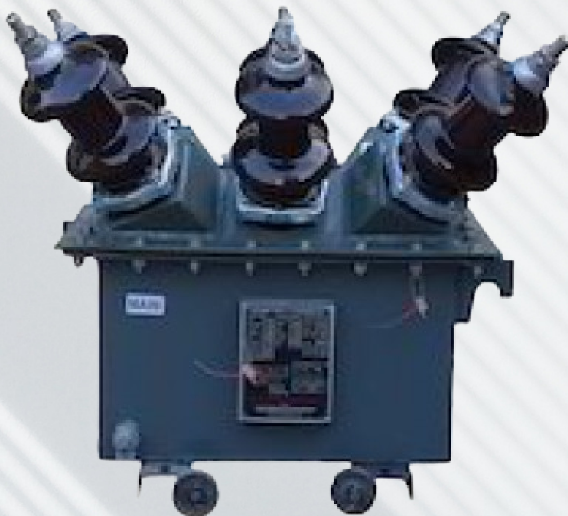
CT PT Combined Metering Unit
